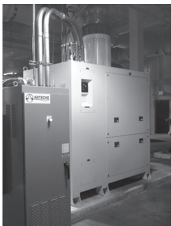
Marine Park WWTF blower
