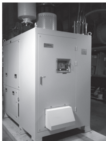
Westside WWTF blower
