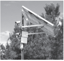
Solar-powered security camera
